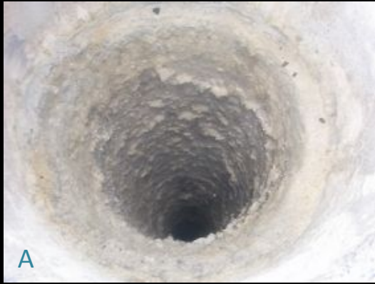
煙突A-E: 劣化度II
