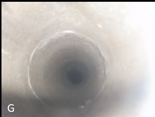
煙突G: 劣化度I
